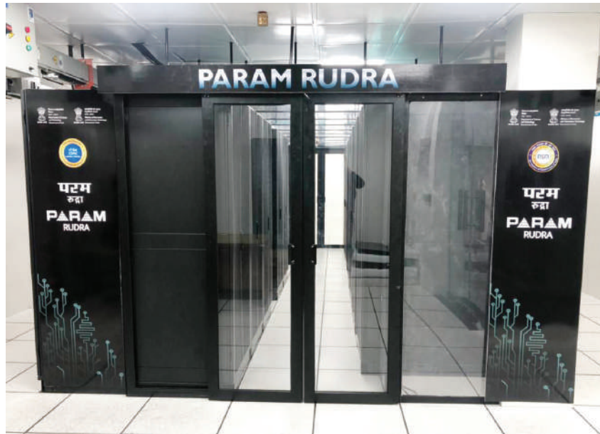
Fig.: 3.1 PetaFlop system commissioned at IUAC, Delhi
