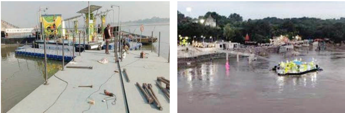
Fig.: World's first floating CNG filling station at Khirkiya Ghat Varanasi (U.P)
