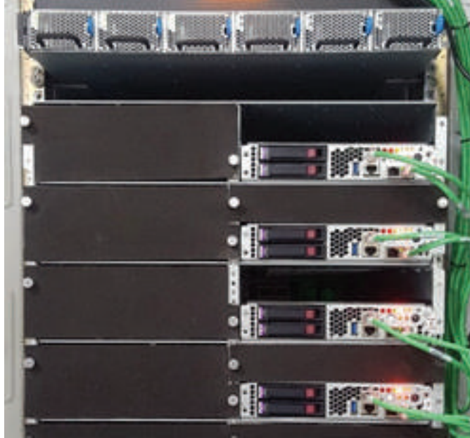
Fig.: Rudra server installed in the rack
