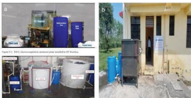
Fig.: (a) 550 L electrocoagulation treatment plant installed at IIT Roorkee (b) 1000 litre Pilot scale at Netaji Subash Chandra Bosh School Hostel, Kunja Bhadur Roorkee.
