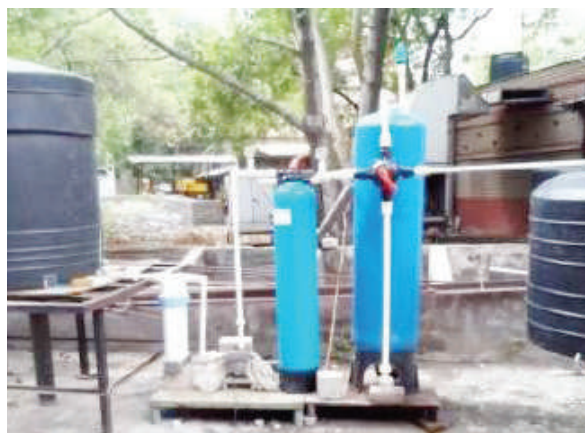
Fig.: Arsenic-removal filter
